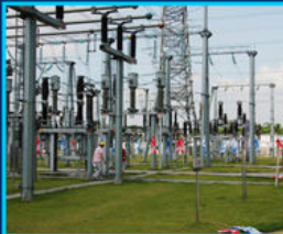
Power Station energy storage
